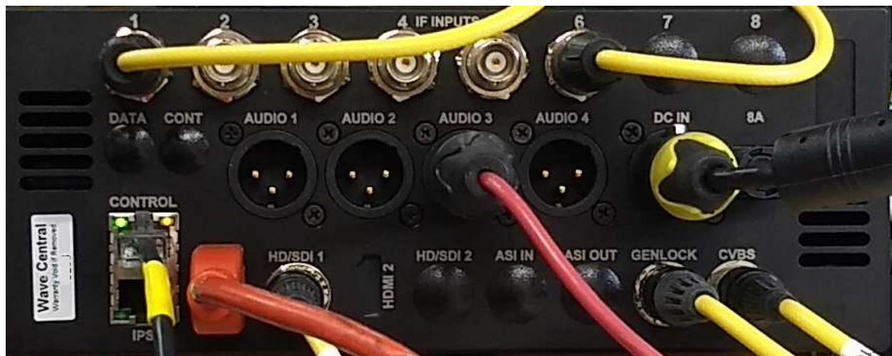
Rear panel as configured for testing
